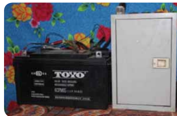
Battery and controller for solar home system.
